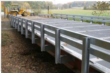
Taking just two days to set the composite panels in place and bolt them to the steel beams, the deck was ready for paving on the third day.
