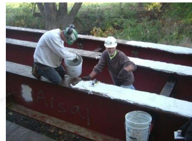
Workers apply thick sand filled epoxy to steel beams to create a leveling bed for the FRP deck panels.
